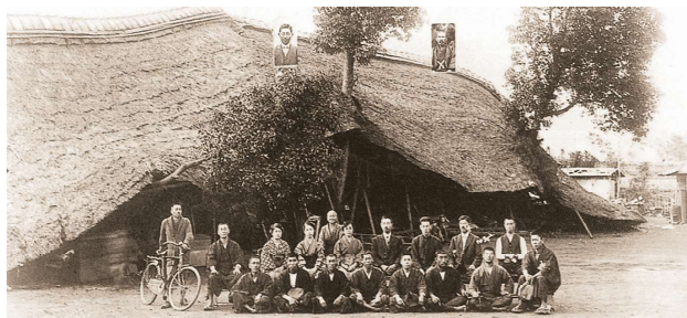
関東大震災で被災した井ノ口尋常小学校 Inokuchi Elementary School, damaged by the Great Kanto Earthquake
